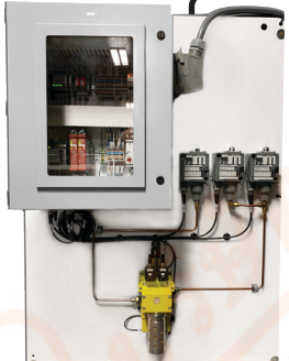
Pneumatic Isolation Panel (PIP)
