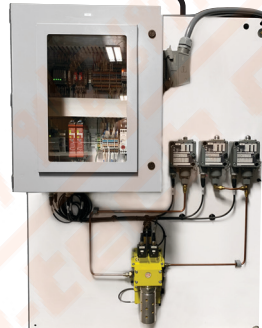
Pneumatic Isolation Panel (PIP)
