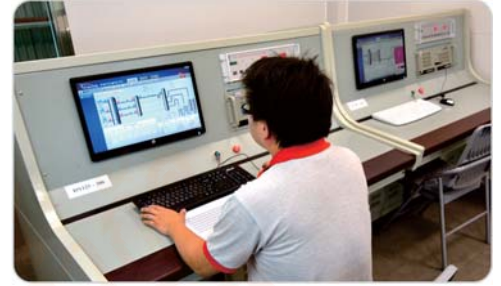
Control room & Graphical HMI
