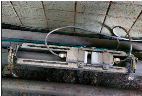
Food industry – pure water boiler pipe
