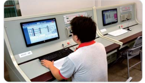
Control room & Graphical HMI
