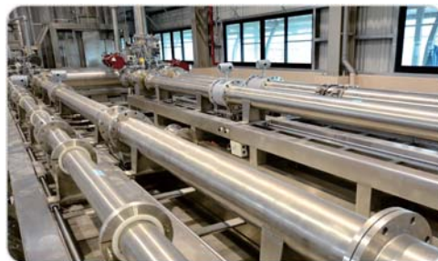
Piping system II (Maximum diameter is 300mm)
