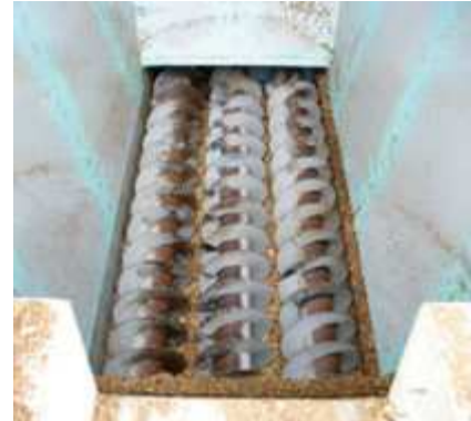
Mounting in discharge screw (wood-fired power plant)
